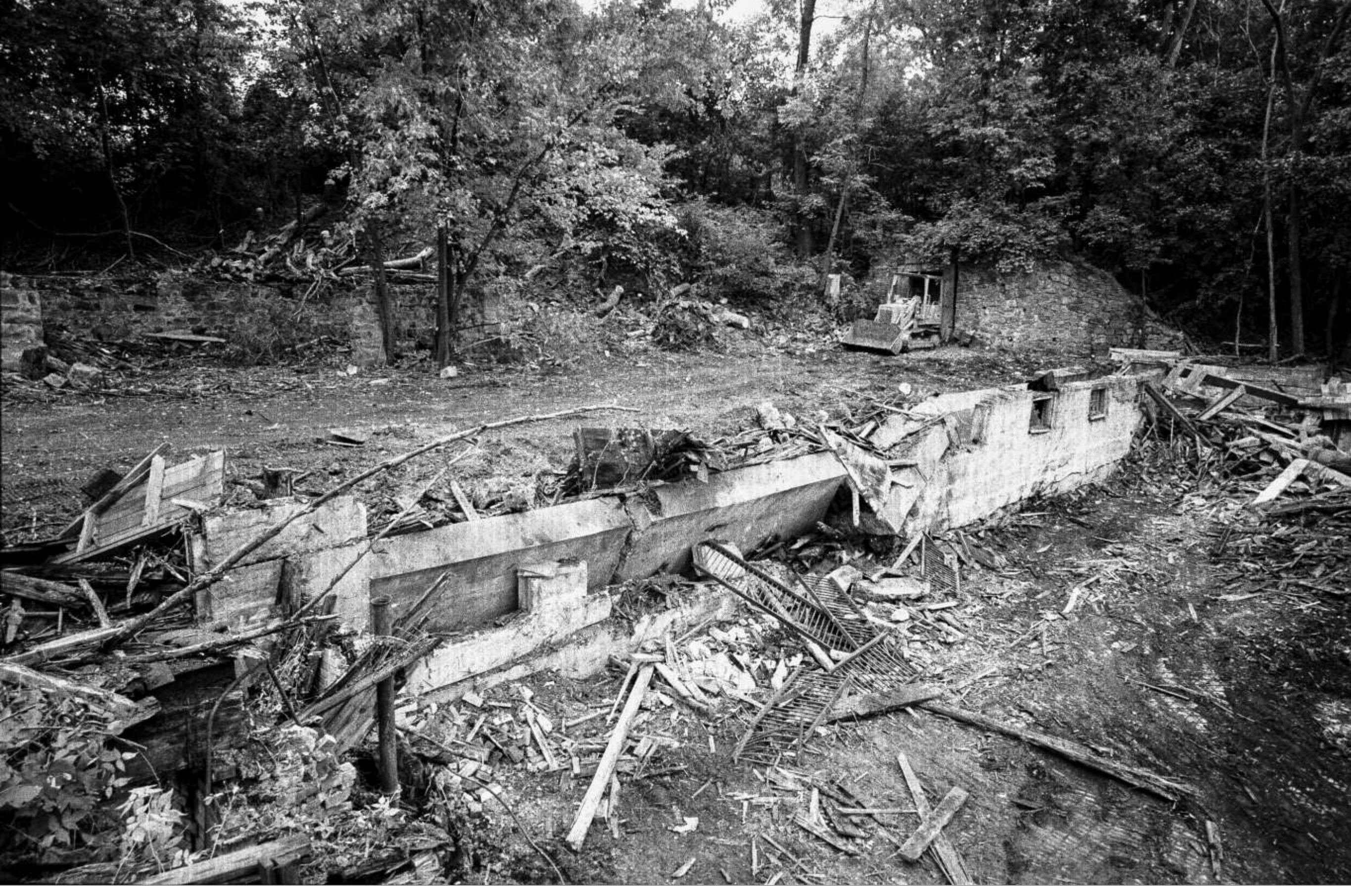
Behind the bulldozer, upper right, is a root cellar buried into the hill. These were common in those days. In the upper left there were more structures probably for the storage of wagons or carriages.
