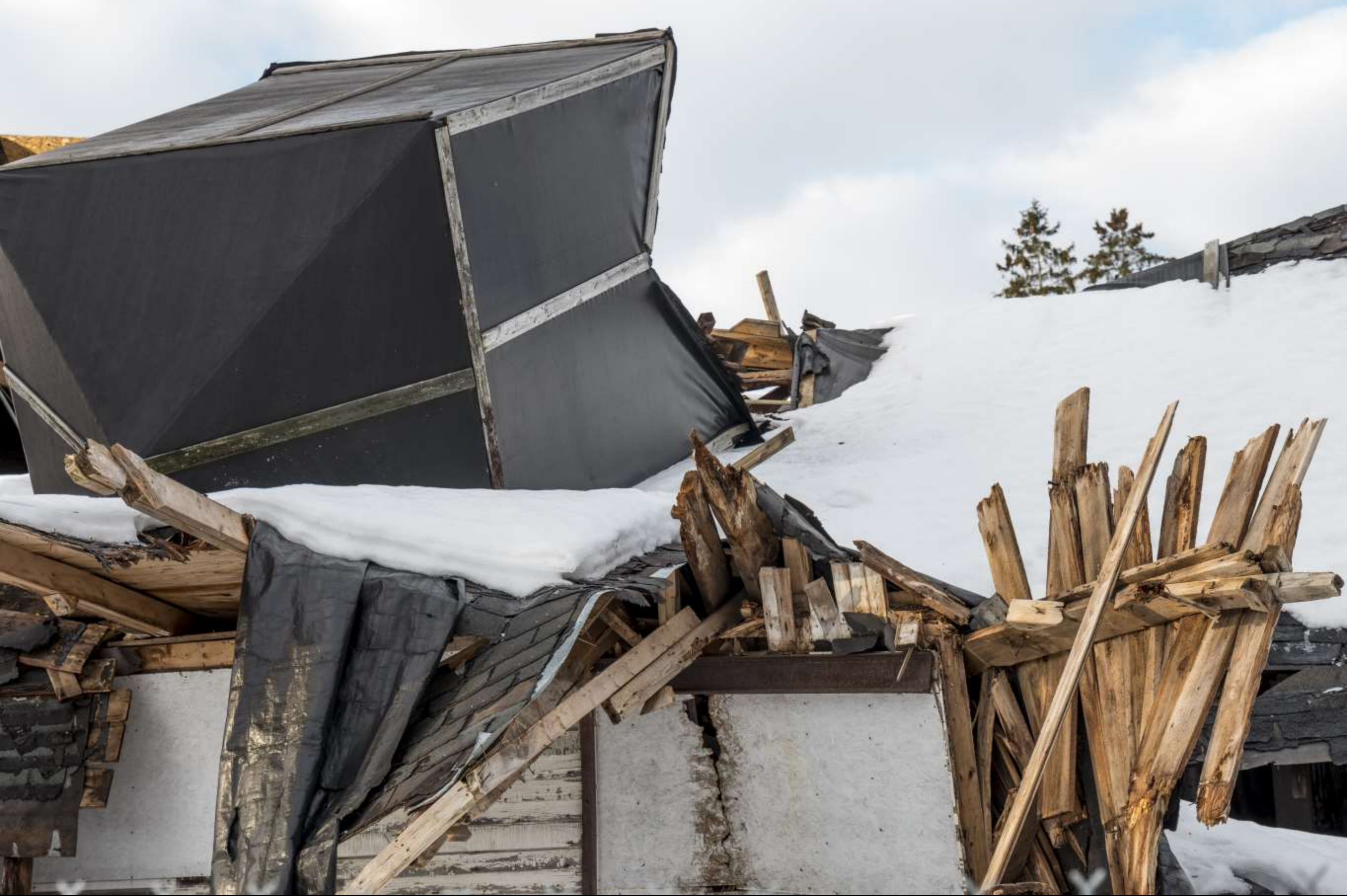
The massive roof vent has toppled over. The bits of wood look like the spine of some huge
