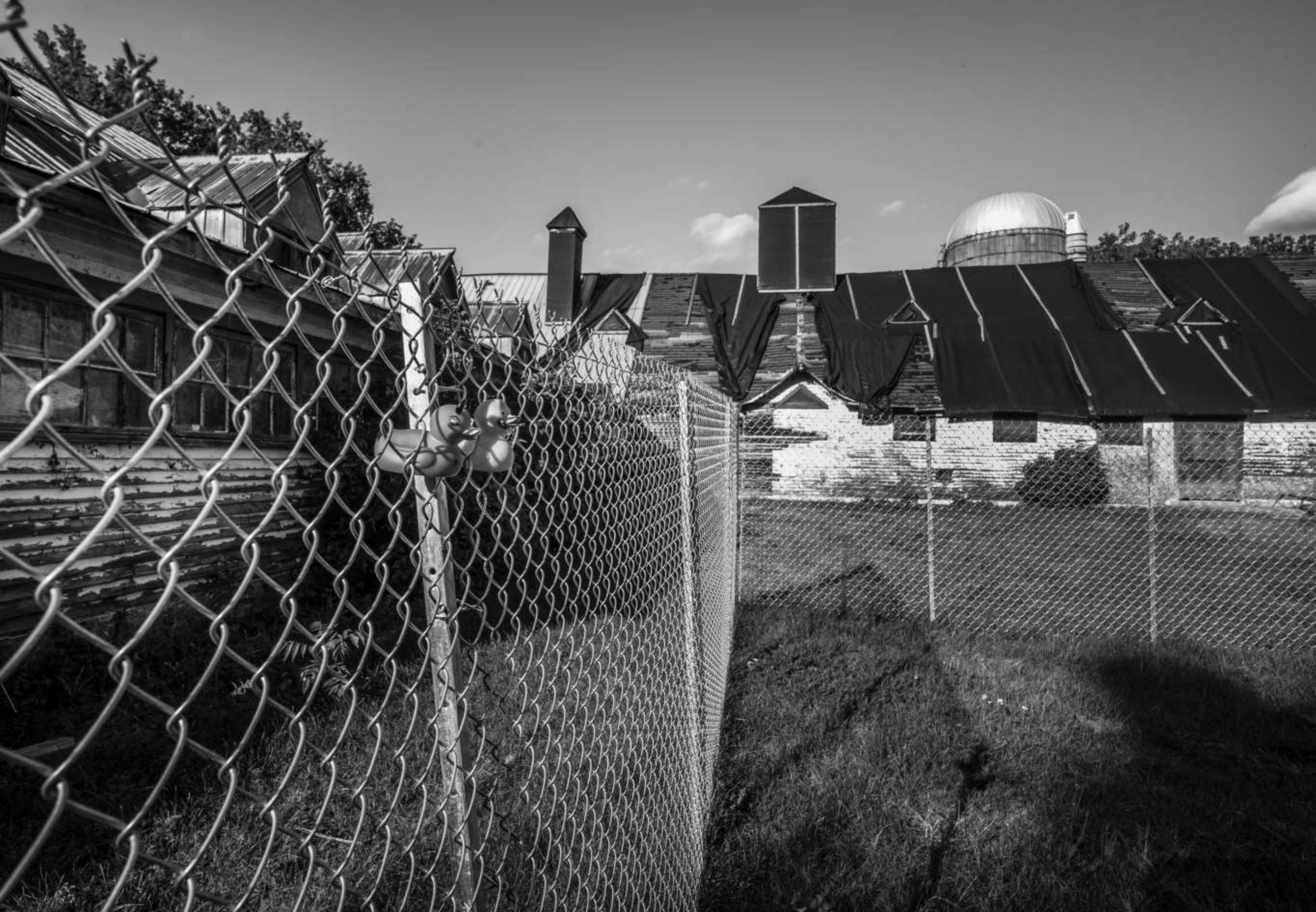
The protective plastic covering has come loose in places. It is possible that the securing nails were driven into wood that was already starting to rot, and they simply did not hold
